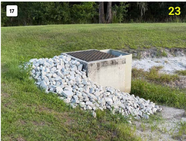
Pond 23 water control structure rip-rap Installation of 2 tons of rip rap to armor the structure from erosion.
