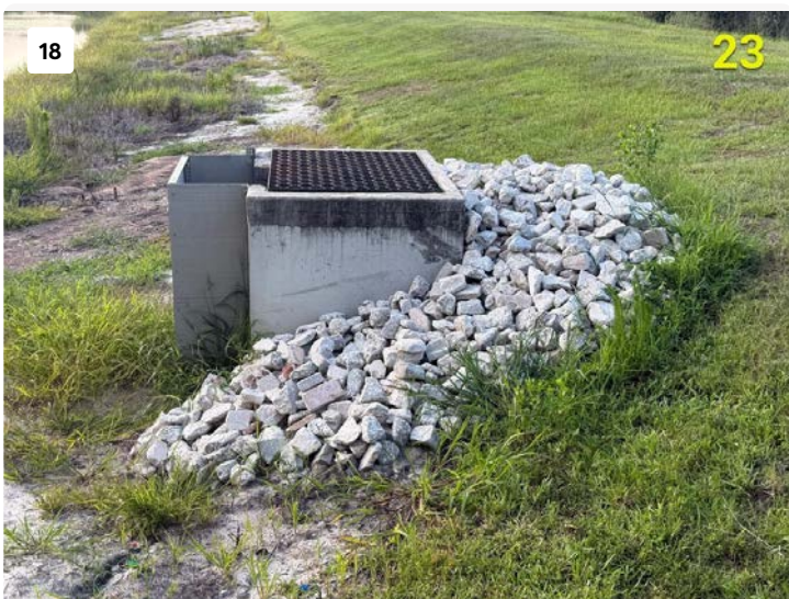
Pond 23 water control structure rip-rap Installation of 2 tons of rip rap to armor the structure from erosion.
